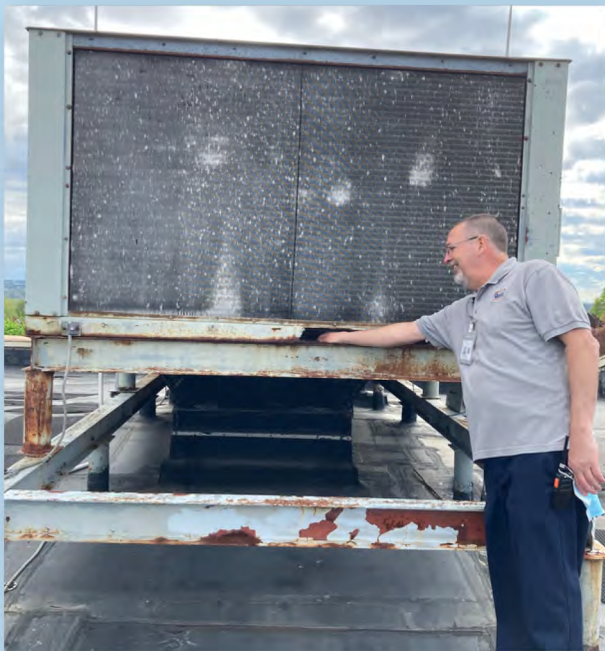
Maintenance Supervisor John Williams puts his hand through one of the HVAC units on the Beth Shalom roof
